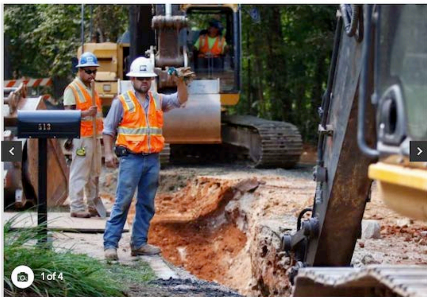
A workman for Moffat Pipe Inc. out of Wake Forest, NC signals a large excavator digging a narrow but deep trench under Hertford Street in the Country Club Hills neighborhood Friday, August 14, 2015. Moffat Pipe is a contractor working for the City of Raleigh to replace older, leak prone terra-cotta sewer lines with new larger 8-inch ductile iron sewer pipes before sewage leaks become chronic. HARRY LYNCH HLYNCH@NEWSOBSERVER.COM
